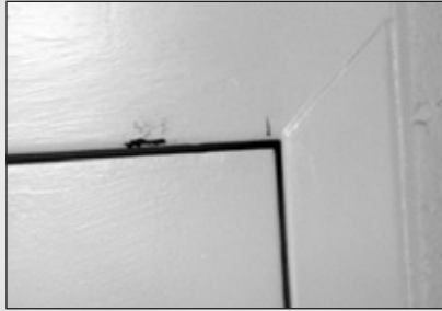
11. The door has similarly moved about 1/8" closer.
